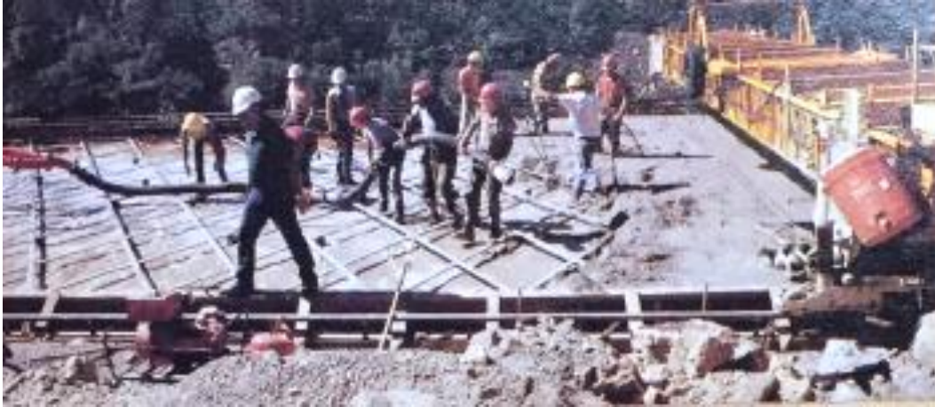
Figure 21. 1986 view of crews installing post-tensioned concrete roadway with steel cables crisscrossed at 45-degree angles. 120
