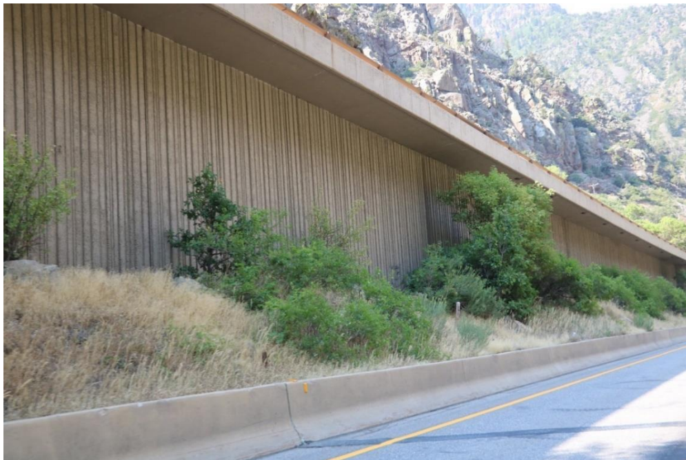
Figure 30. View of retaining wall with textured concrete panels featuring vertical grooves. Mead & Hunt, Inc. photograph.
