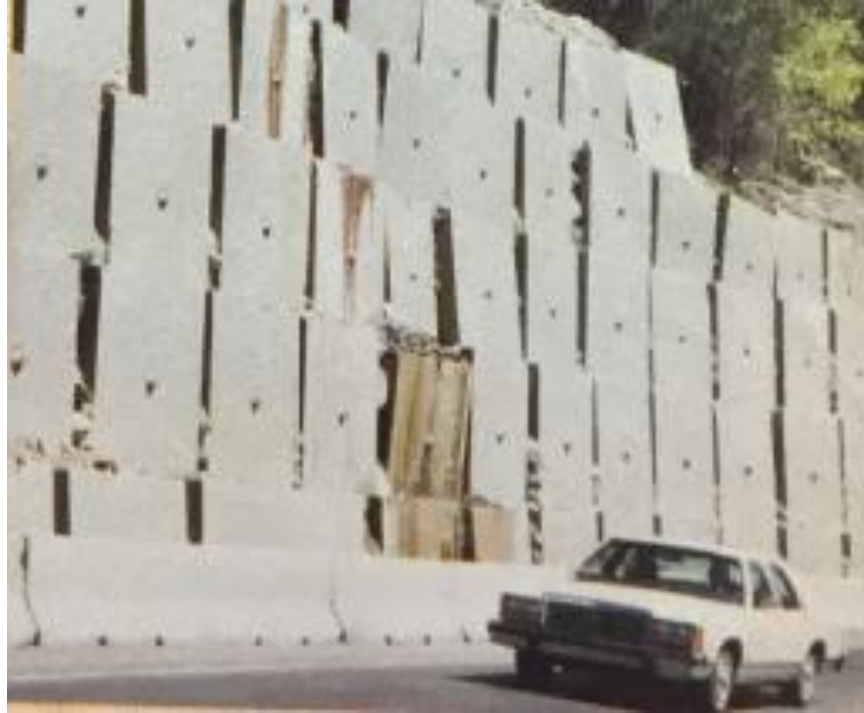
Figure 27. Temporary pre-cast retaining walls installed along the highway in 1986 in preparation for construction of permanent retaining walls. 130
