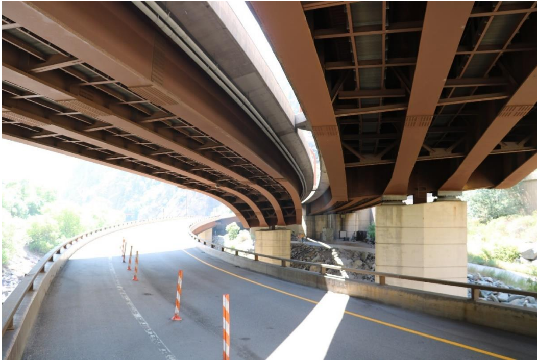
Figure 17. Welded steel plate girders enabled the structure to curve in order to follow the contours of the canyon wall and Colorado River. Mead & Hunt, Inc. photograph.
