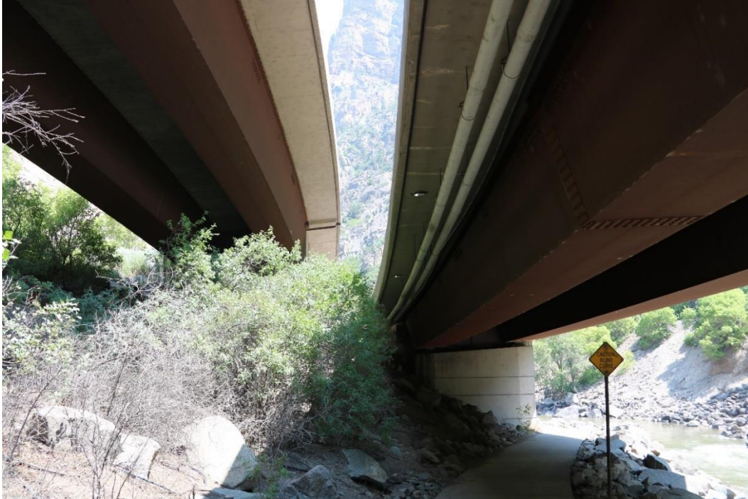
Figure 15. View of twin steel box girders near the Shoshone Rest Area. Mead & Hunt, Inc. photograph.
