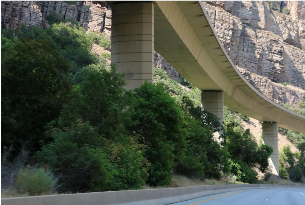
Figure 19. Segmental concrete box girder located just west of Reverse Curve Tunnel, view facing northeast. Mead & Hunt, Inc. photograph.
