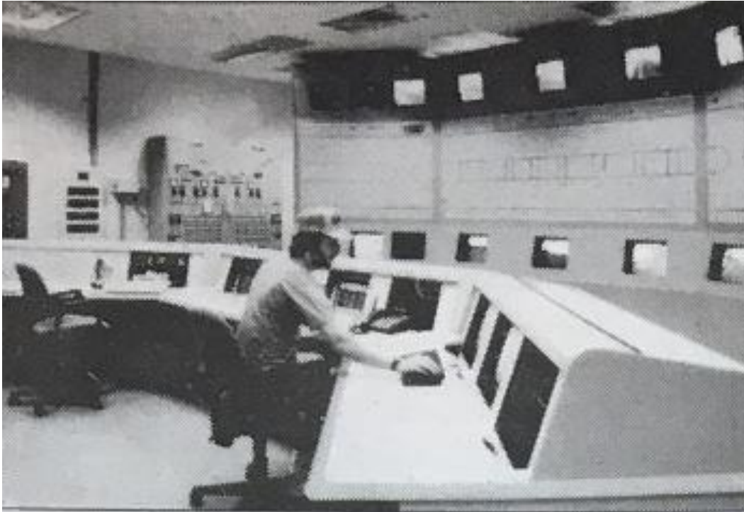
Figure 25. View of centralized control center within the Hanging Lake Tunnel structure, which was state-of-the-art at the time. 126
