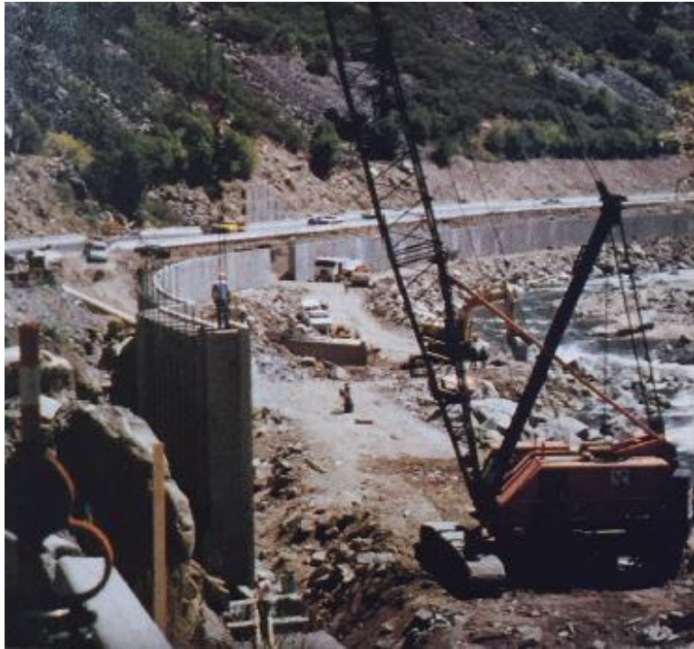
Figure 29. Construction crews install retaining walls that consist of T-section concrete panels to support the upper roadway and to retain earth. 136
